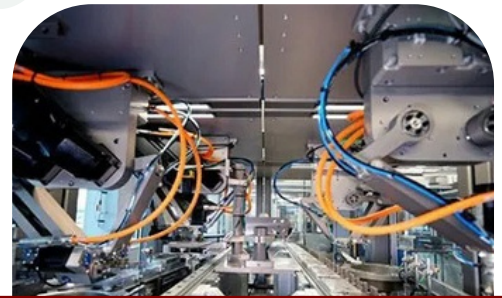
ATS System Programming & Installation – Prince Abdullah Hospital, Bisha
