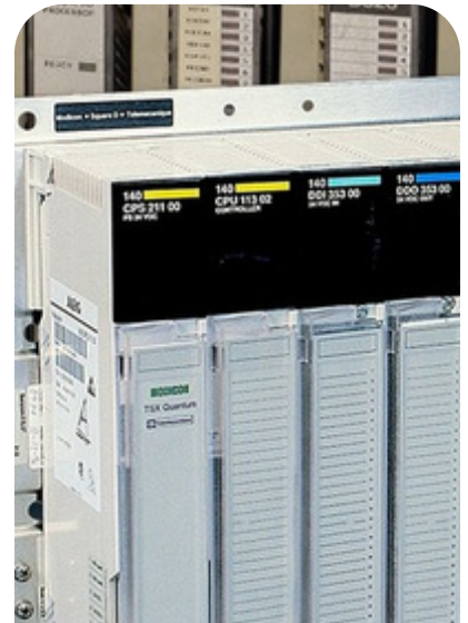
Modicon PLC Upgrades – Jeddah Beverage Can Making Co. (JBCMC)
